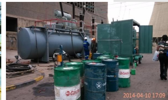
ZPC Hwanqe Power Station, Zimbabwe.
